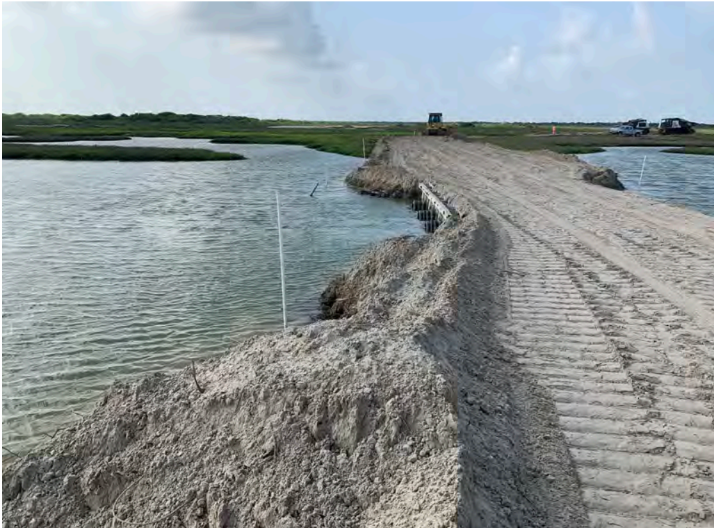
Photo 11. East side of levee raise and breach repair at CD-SR-1 (looking south). Side slopes have not been placed and reclaimed material topping not placed.
