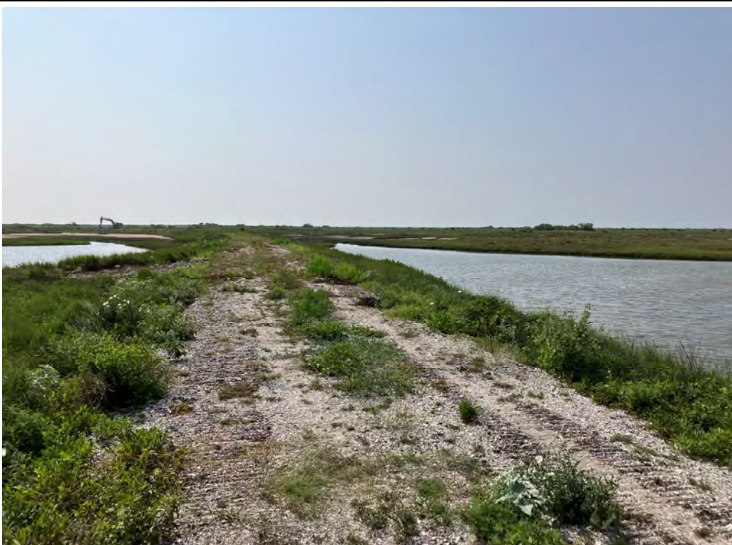
Photo 6. Existing condition of east berm roadway approach of FH-SR-3 site (looking east)
