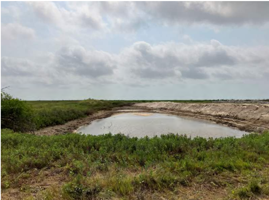
Photo 10. Water feature that will expand as sediment source for FH-SR-3. Some stripping and grubbing along eastern shoreline.
