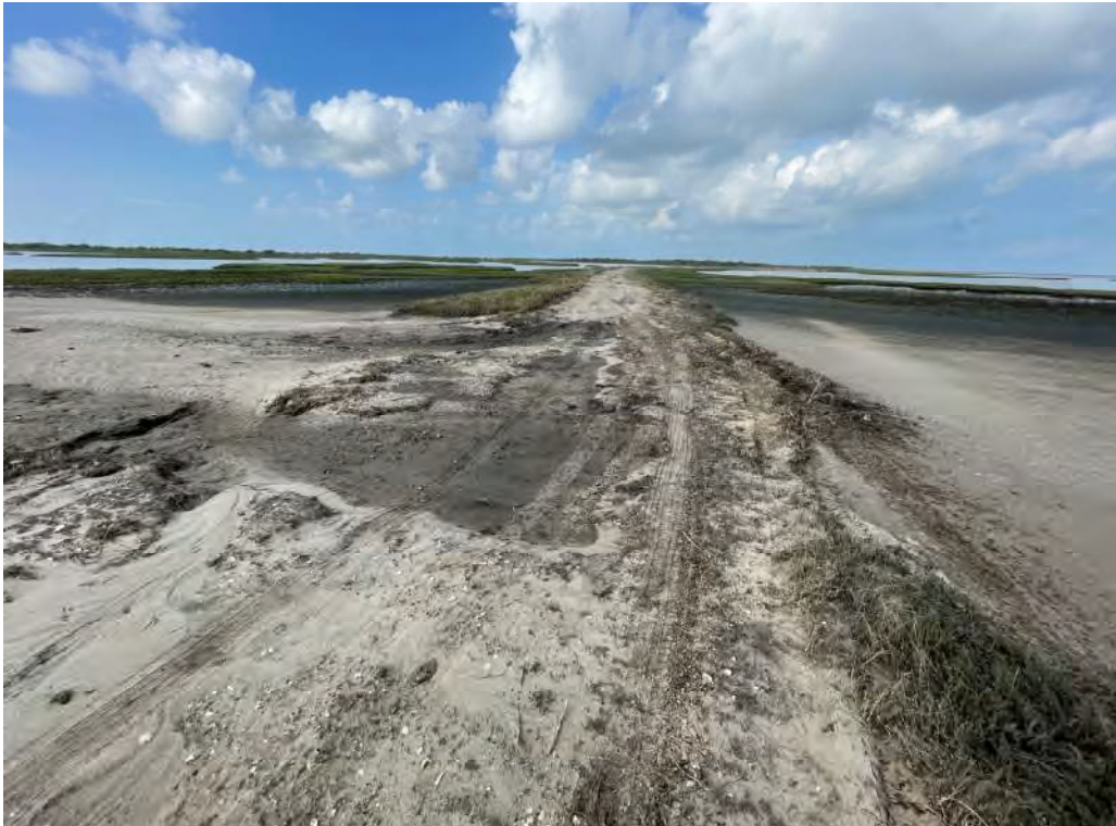
Photo 2. Roadway washout caused by Tropical Storm Alberto between B-SR-1 and BC-SR-1 sites.
