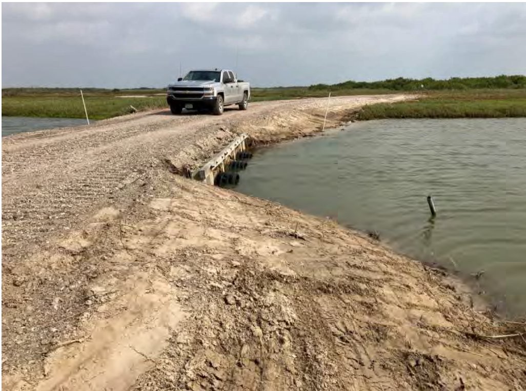
Photo 8. East side of levee raise and breach repair at CD-SR-1 (looking north). Side slopes have been graded and reclaimed material topping placed.
