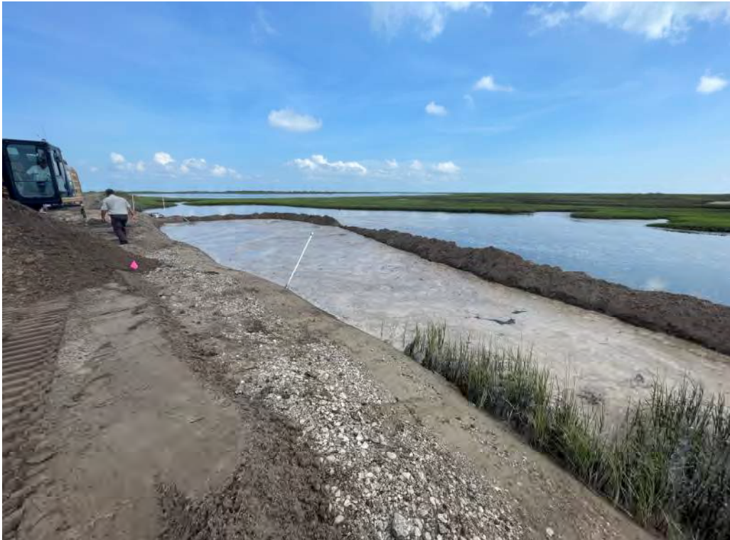
Photo 10. Pumping water out of site to prepare for side slope repair on FH-SR-3 (facing west)
