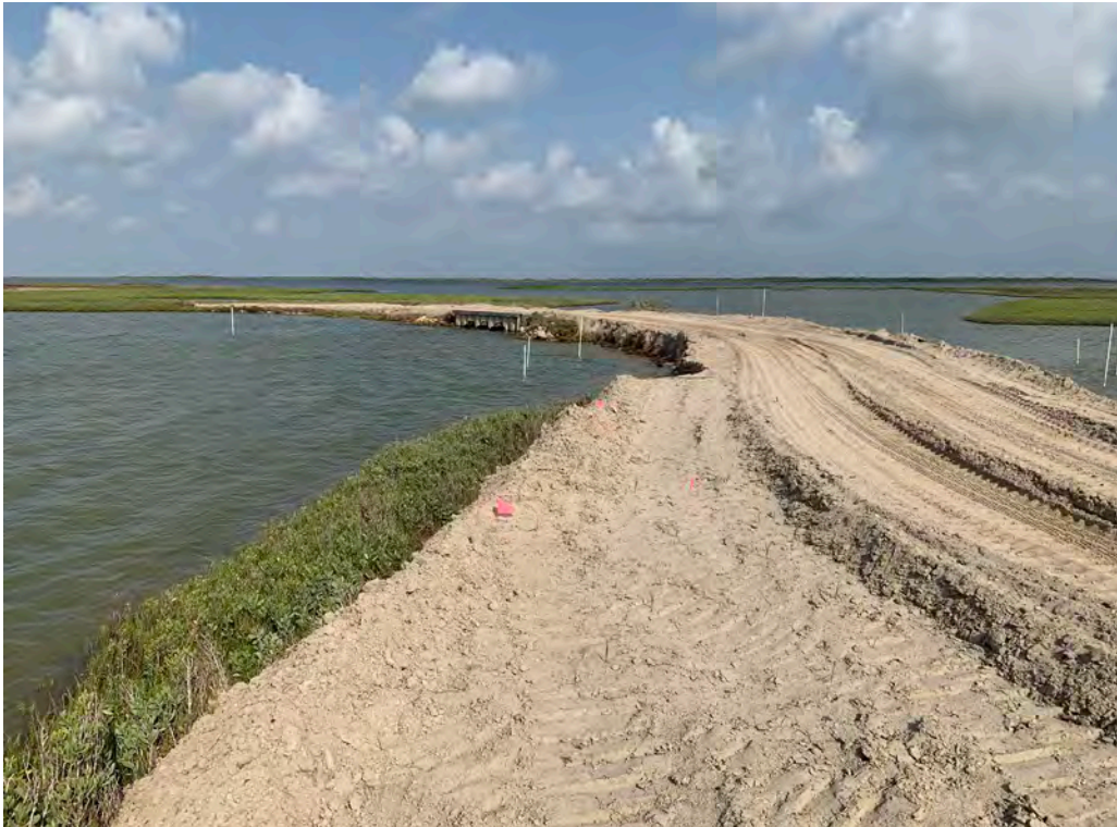
Photo 5. Southern shoreline of BC-SR-1 approaching breached area (looking west). Note side slope not placed. Also can see scarping of material from waves in Little Brundrett Lake.
