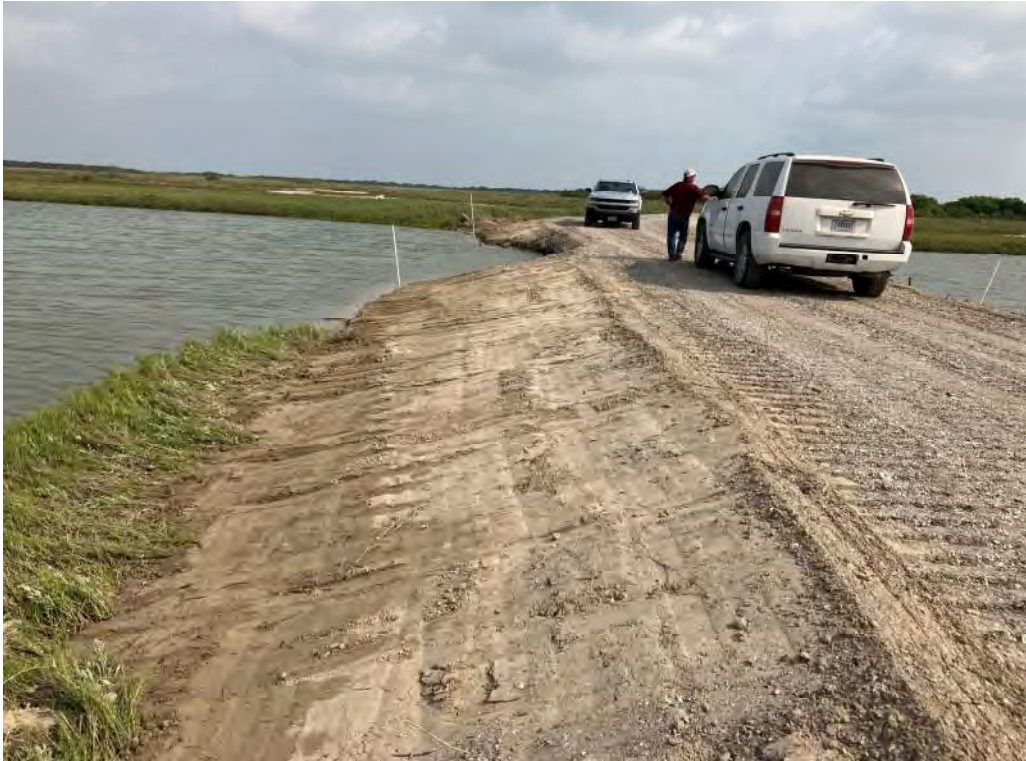
Photo 7. West side of levee raise and breach repair at CD-SR-1 (looking north). Side slopes have been graded and reclaimed material topping placed.
