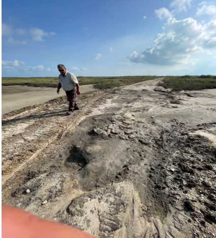
Photo 1. Roadway washout caused by Tropical Storm Alberto between B-SR-1 and BC-SR-1 sites.
