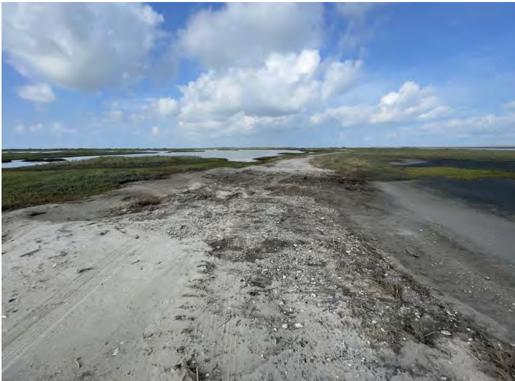
Photo 3. Roadway washout caused by Tropical Storm Alberto between B-SR-1 and BC-SR-1 sites.
