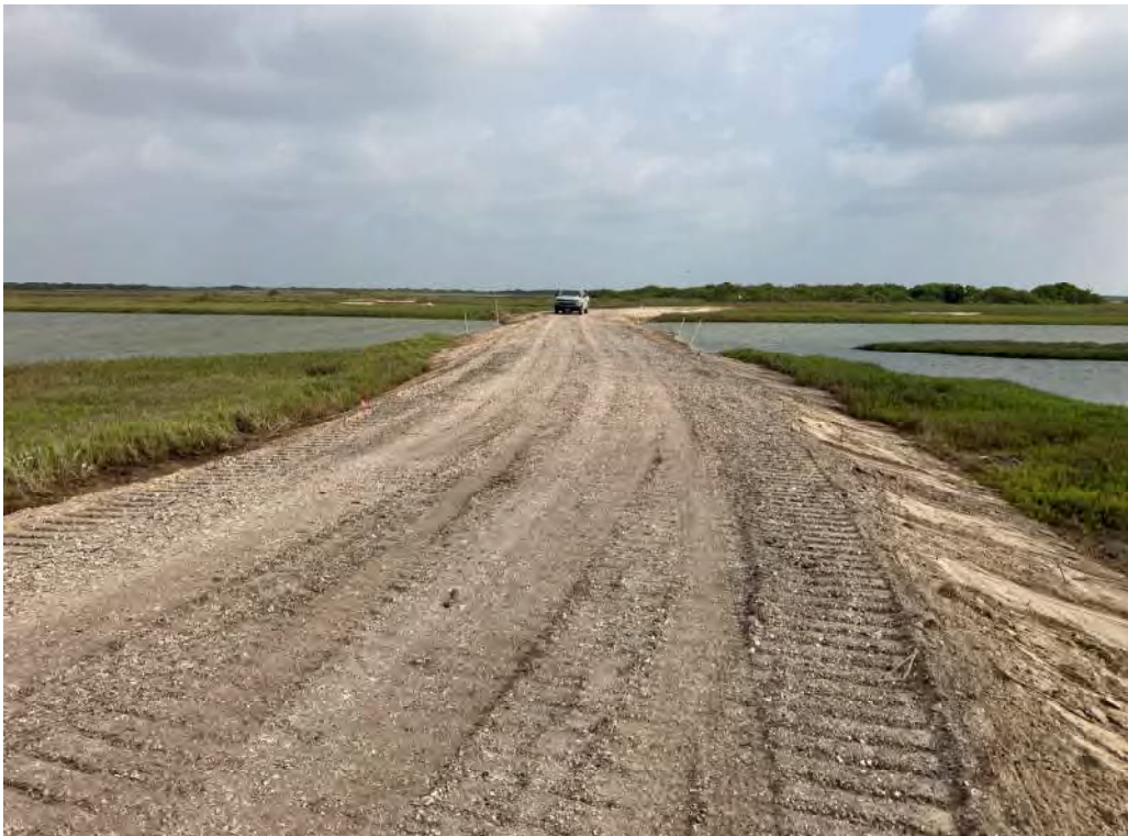
Photo 6. Breach repair at CD-SR-1 (looking north). Side slopes have been graded and reclaimed material topping has been placed.
