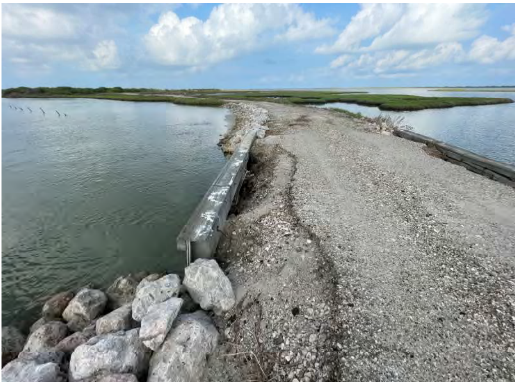
Photo 5. BC-SR-1 structure wash out (looking west).
