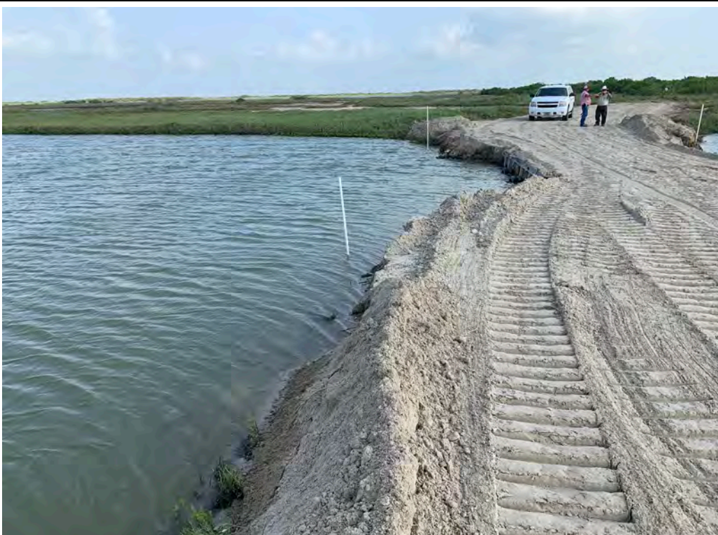
Photo 12. West side of levee raise and breach repair at CD-SR-1 (looking north). Side slopes have not been placed and reclaimed material topping not placed.
