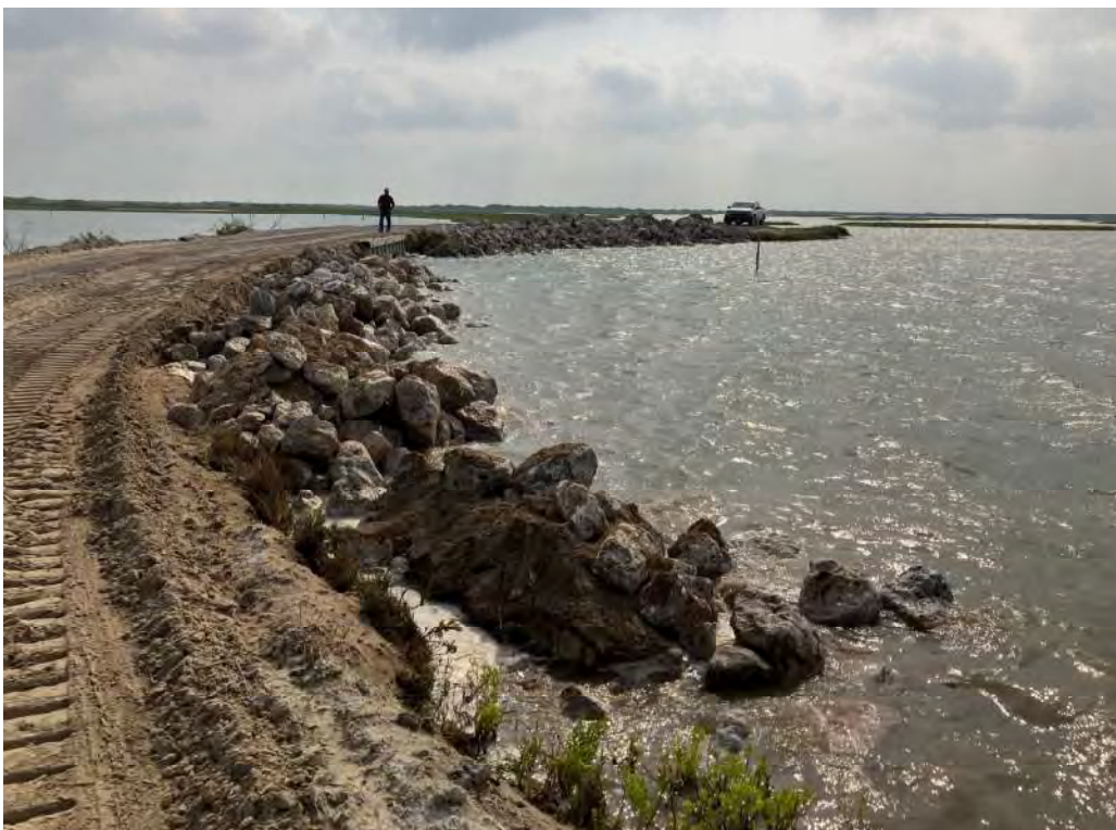
Photo 4. Rock rip rap placed along southern shoreline on western end of BC-SR-1 (looking east)
