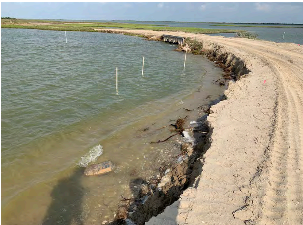
Photo 6. Southern shoreline of BC-SR-1 at breached area (looking west). Note side slope not placed. Also can see scarping of material from waves in Little Brundrett Lake.
