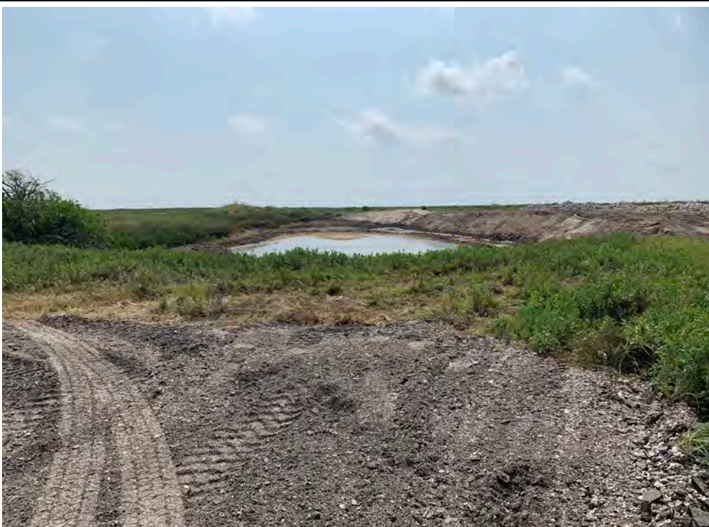
Photo 14. Water feature that will expanded as sediment source for FH-SR-3. Some stripping and grubbing along eastern shoreline.
