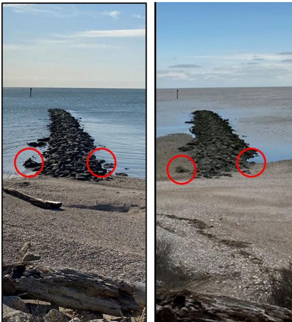
Figure 7. Terminal groin of Schicke Point living shoreline constructed in April 2017. Image on left taken on January 11, 2022. Image on right taken March 17, 2023. Red circles include rocks visible in both photos. Water level at Port Lavaca on January 2022 was 0.58 feet higher than on March 17, 2023. Water level at Port O'Connor was 0.15 feet higher on March 17, 2023 than when the photo was taken on January 11, 2022.
